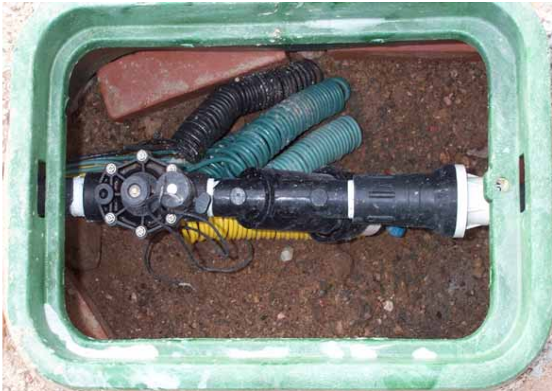
A typical valve assembly. The water source is located on the left, with water flowing through the assembly toward the right.
